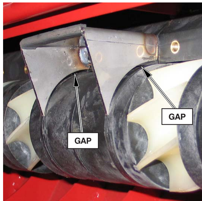
Incorrectly Installed Blank Off
